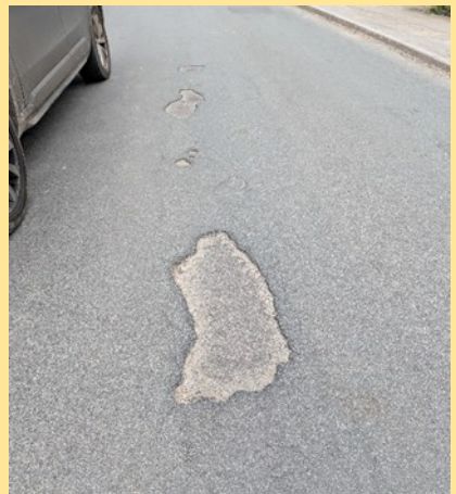
Deteriorating surface on Old Alexander Road
