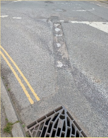
Eroding utility repairs Gloucester Road (we had loads to choose from)
